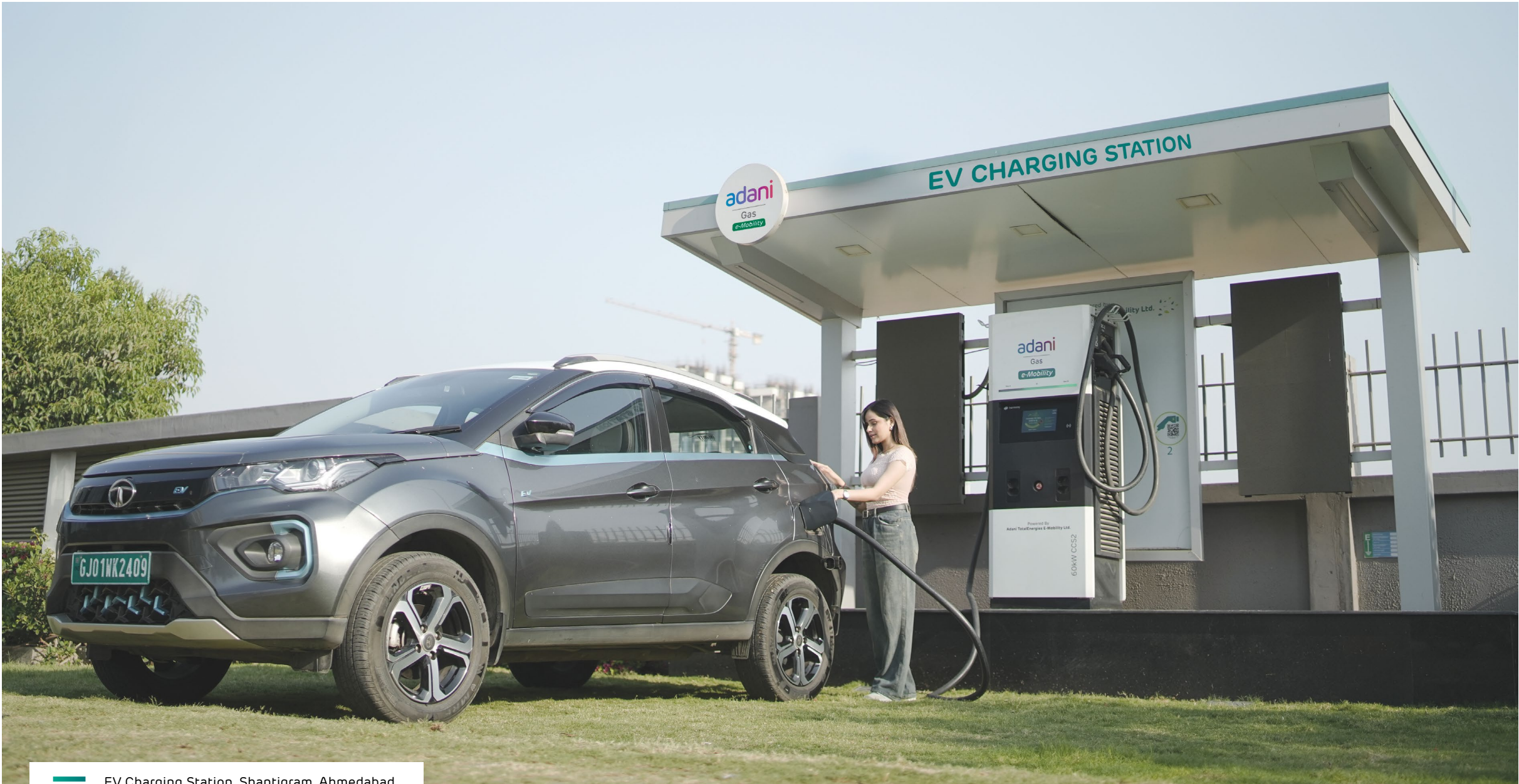
EV Charging Station, Shantigram, Ahmedabad
